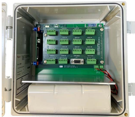
Inside Data Logger Enclosure
